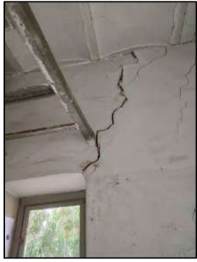
crack above the window
