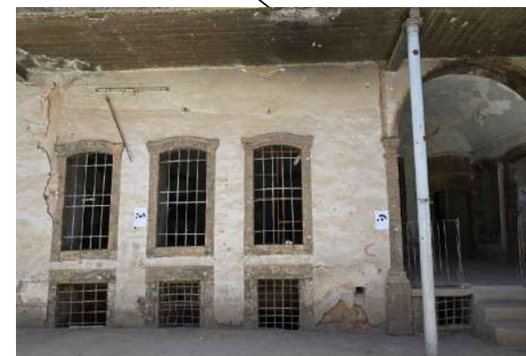
The cracks in the Central courtyard
