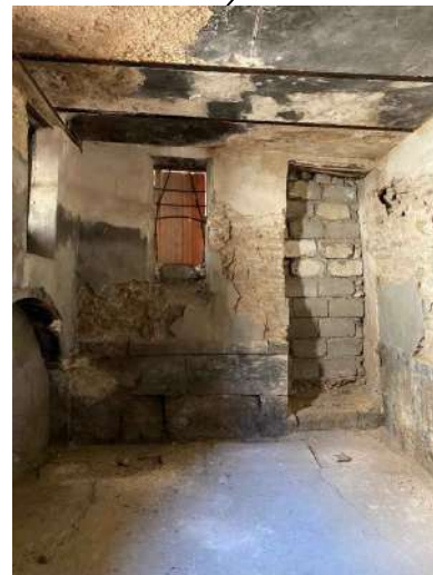
ceiling had loss of masonry and cracks due to explosion near by
