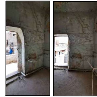
moisture coming from the roof and it is affecting the wall
