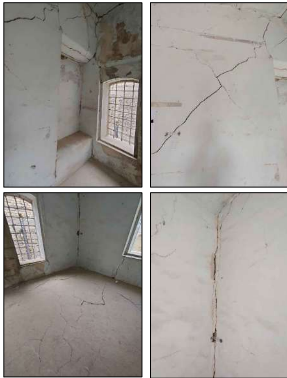
this is the most dangerous room in the building it is leaning towards the street and it contains too many cracks ( diagonal cracks , cracks at the corners , cracked floor and cracks above the window ).
