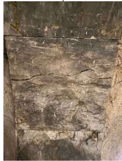
Cracks in the selling of the basement was deep and extends to alabaster
