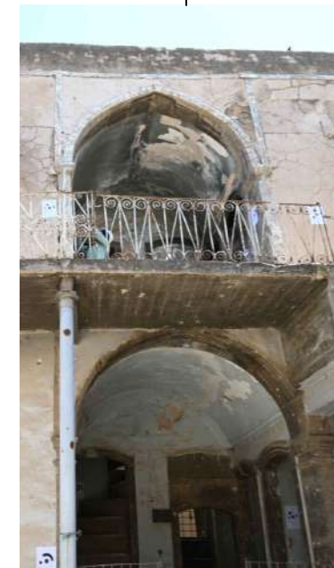
AL-EWAN which is considered as main element in the old house in Mosul
