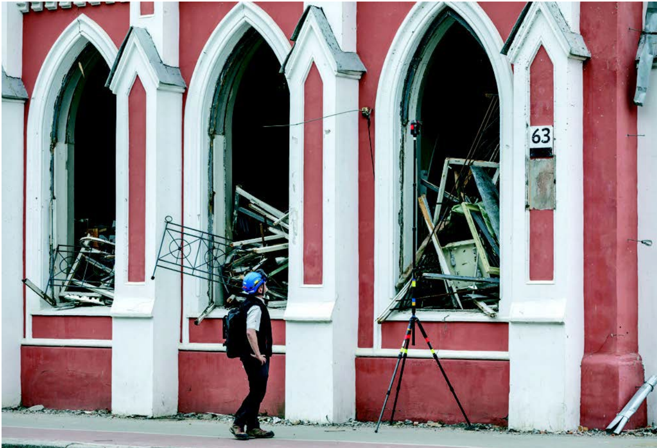
Fieldwork in Chernihiv. Assessing damage to V. Tarnovskyi's historical building in partnership with HERI, ICCROM and ICOMOS teams
